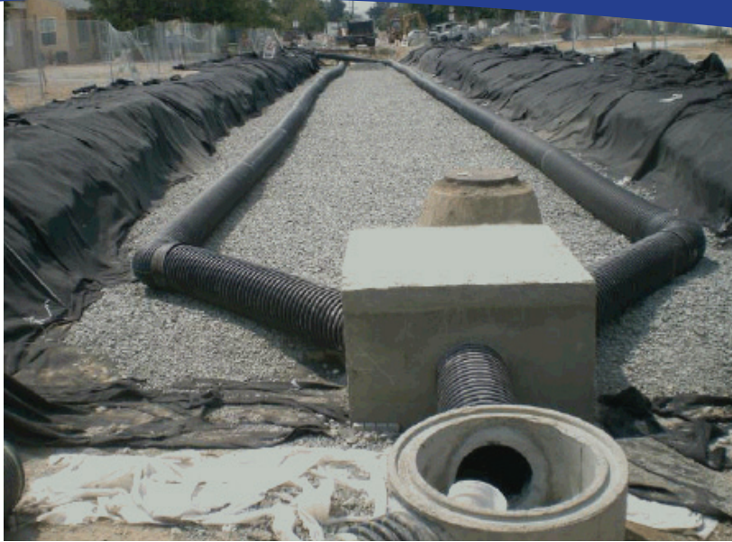
Project Infiltration Gallery
