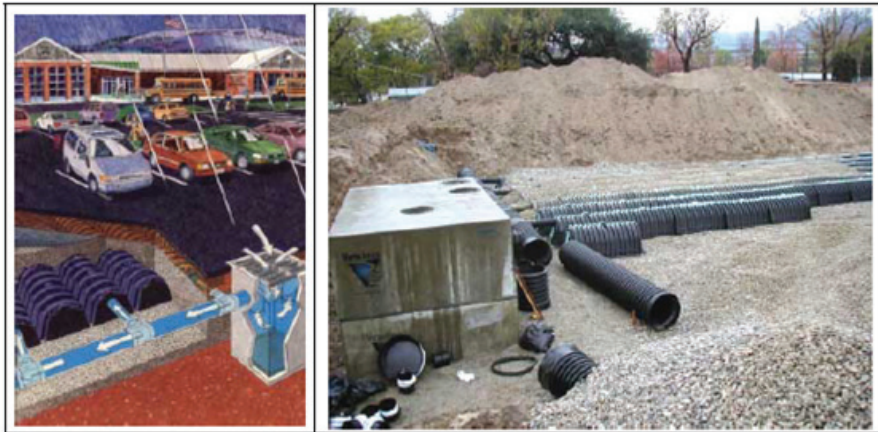
Figure A-4: Parking Lot Infiltration Project
